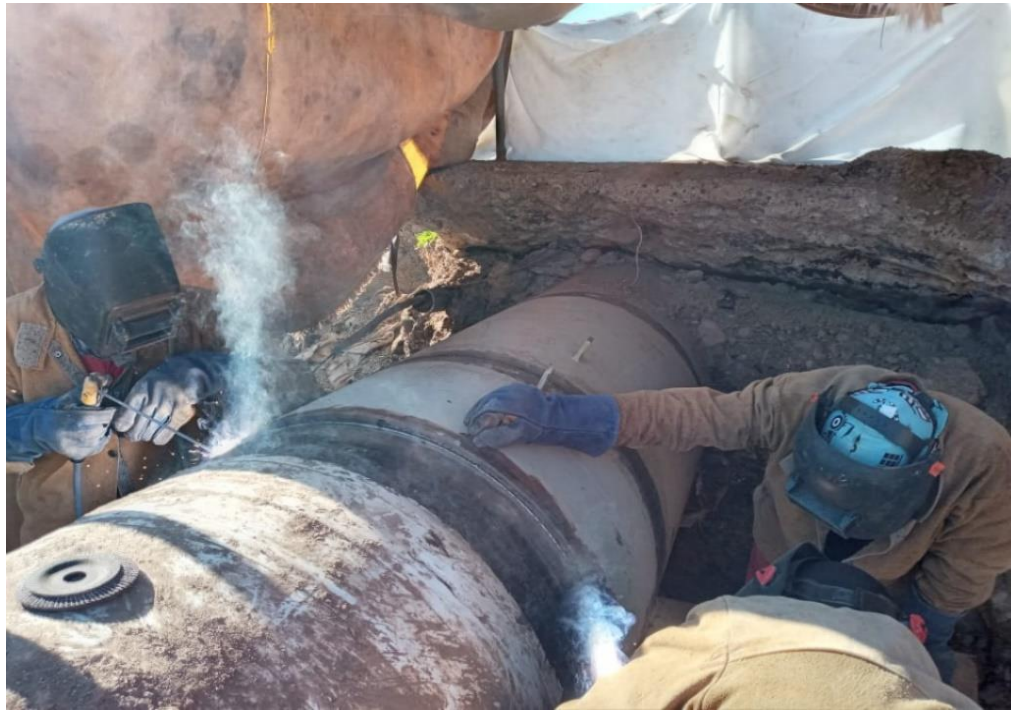
Figure 0-1 Circumferential weld – Sleeve type B is welded directly to carrier pipe-in-operation-36 Inch Kurdistan pipeline- Erbil
